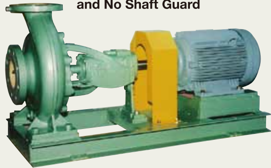
Existing Pump with Standard Coupling Guard and No Shaft Guard
