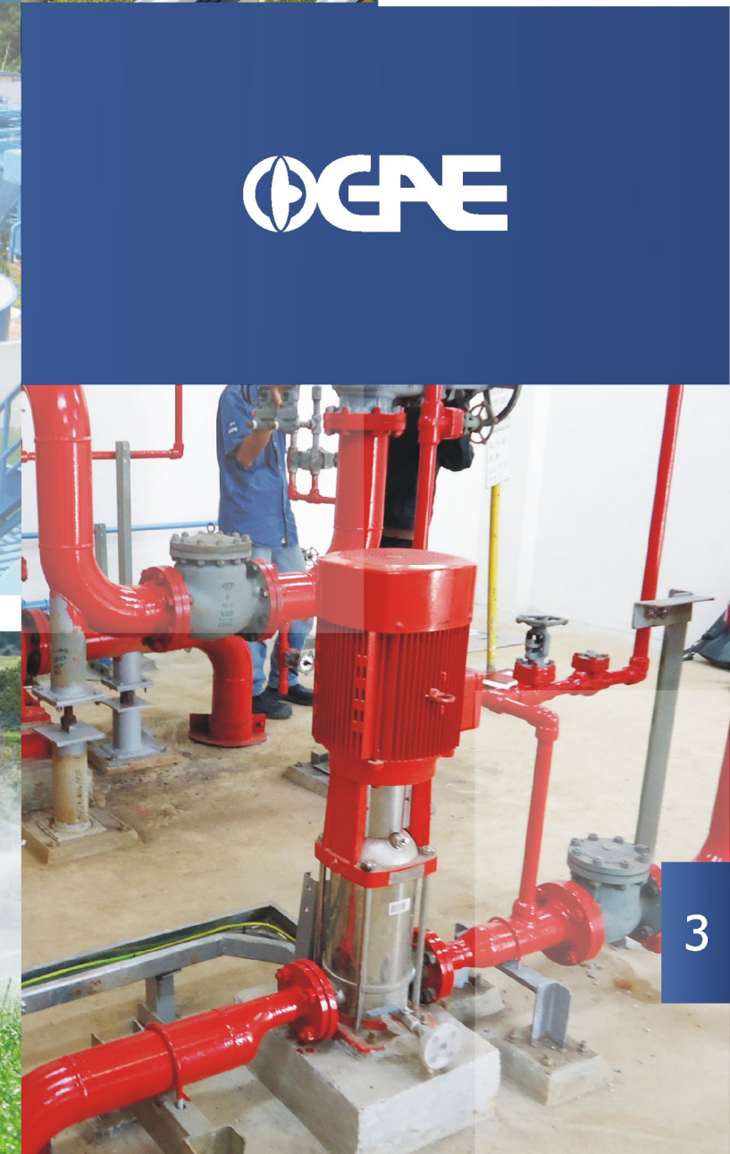
Fire Fighting Systems
